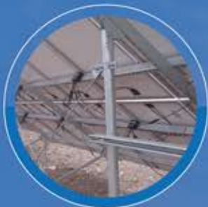
SOLAR MODULE MOUNTING STRUCTURES
